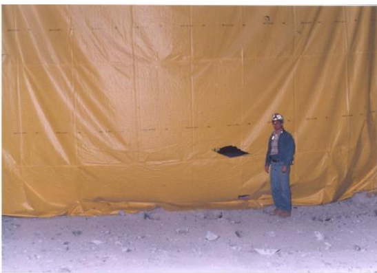
Figure 6. Fly rock damage in brattice cloth.
