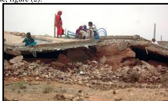
Figure (2): Collapse of buildings even if made of strong building materials
